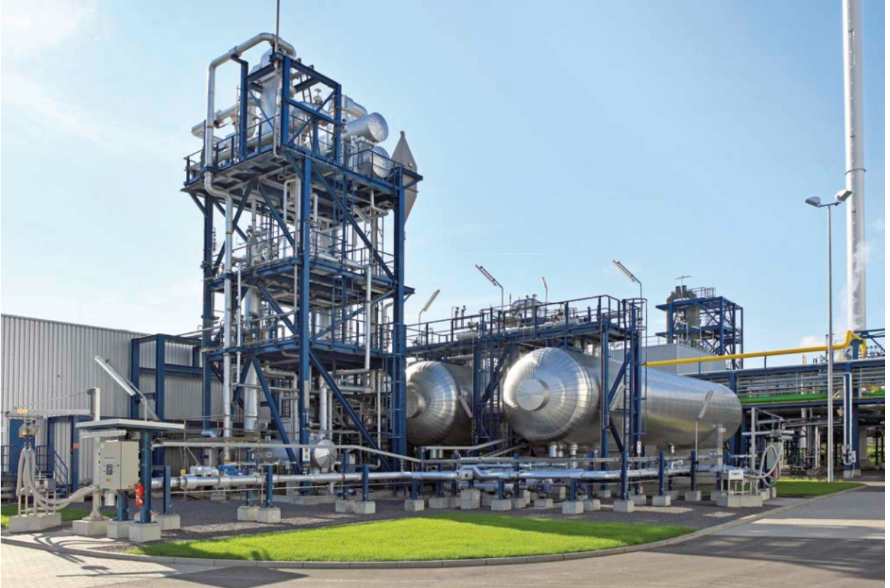
Figure 1: CO 2 plant in Schwarze Pumpe
