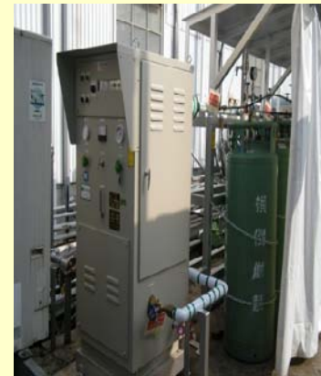
CO 2 supply system (Max.300kg/h CO 2 gas)
