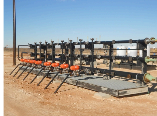
CO 2 injection manifold Courtesy B Hill, Clean Air Task Force
