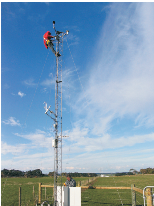
This flux tower being installed at a geologic storage site measures the concentration of gases in the atmosphere. Such devices can detect increases in CO 2 .
