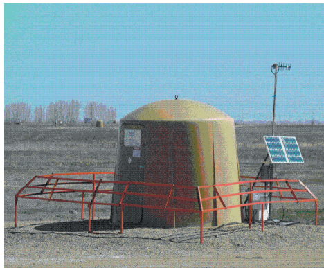
CO 2 Storage Injection Site
