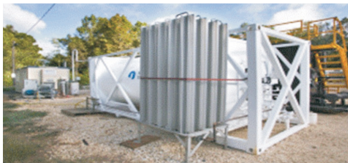
Underground water quality can be monitored for any changes due to CO 2 using specially-designed devices.
