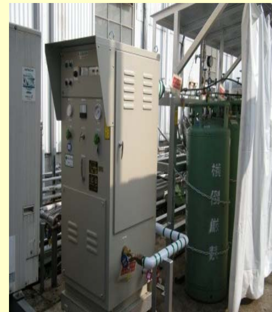
CO 2 supply system (Max.300kg/h CO 2 gas)
