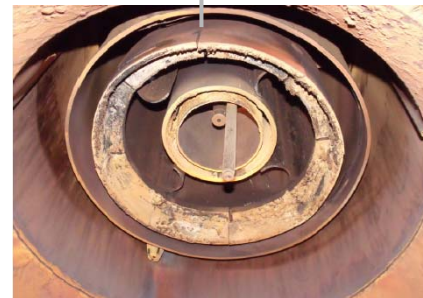
Burner 4: swirl burner as pre-mixed burner
